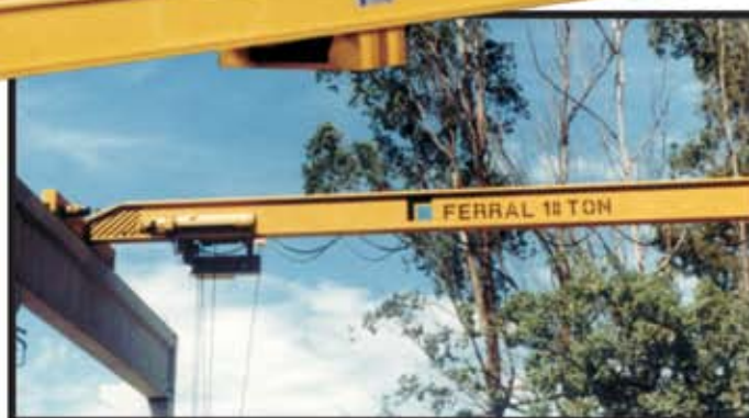
Ponte Rolante 10 t X 20m Travelling Crane 10 t x 20m
